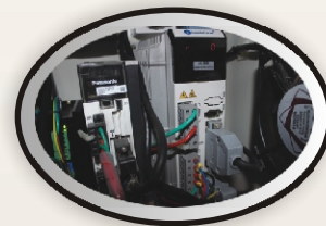
Panasonic Servo driver to run Stainless steel bending roller
